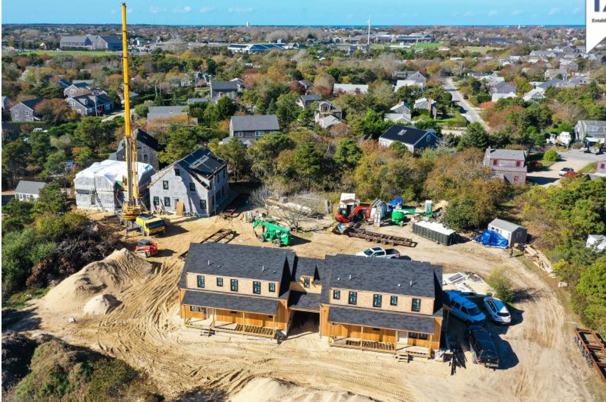
An aerial view of an affordable housing project on Nantucket. The town has dedicated about $70 million to housing going back to 2019. Courtesy of the town of Nantucket
